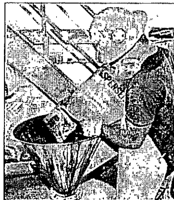
Figure 135 Adzrakmen wearing personal protective equipment, adds dry components to the mud through a hopper.
