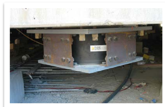
Figura 2.15 Utah State Capitol's Isolator
