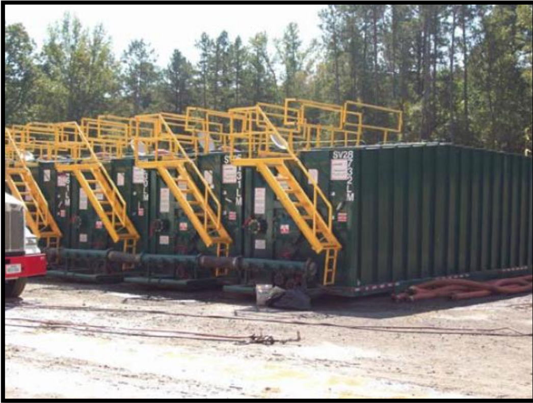
Fig.5.6. Contenedores de agua – Tanques “Frac” en la lutita de Fayetteville (J. Daniel Arthur, SPE, Brian Bohm, Bobbi Jo Coughlin, and Mark Layne, SPE, ALL Consulting, “Evaluating Implications of Hydraulic Fracturing in Shale Gas Reservoirs”, SPE 121038, 2009).
